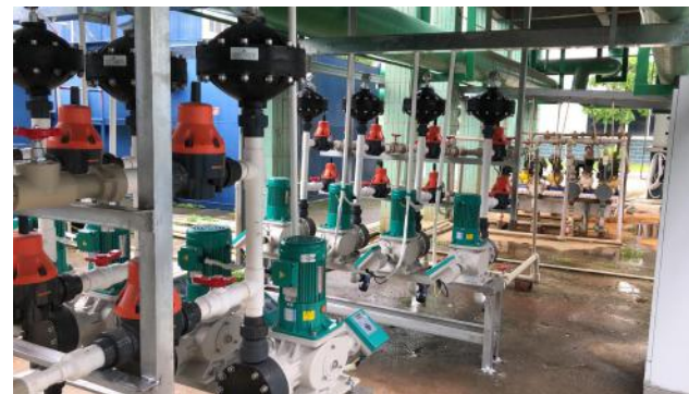
GX · Wastewater Treatment
