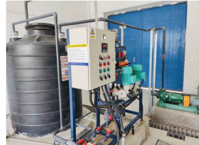
NX · Wastewater Treatment
