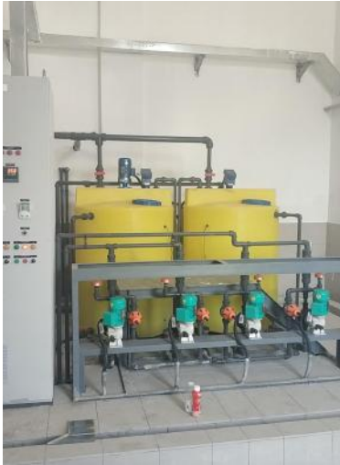
HB · Wastewater Treatment
