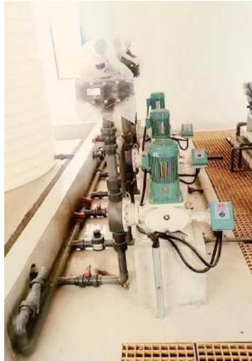
BJ · Water Plant
