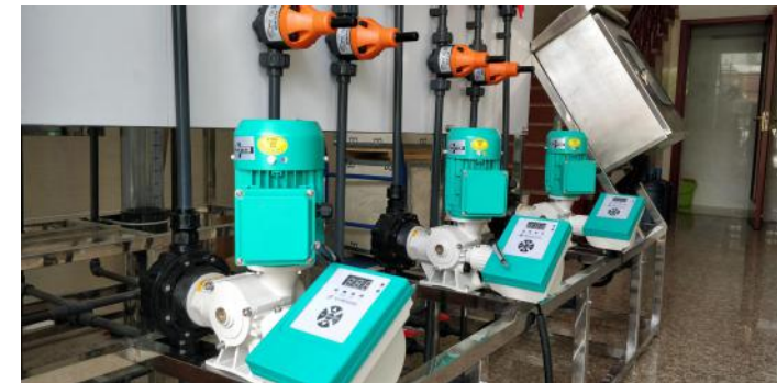
HLJ · Water Plant
